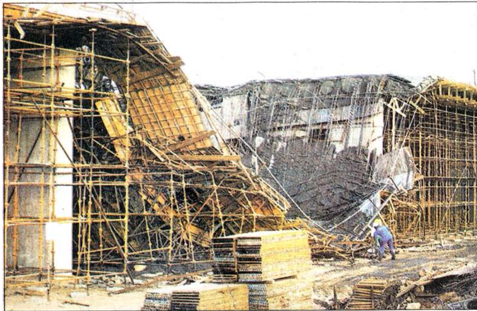
DEADLY LETDOWN: Scenes such as this collapse of Port Elizabeth's Coega Bridge in 2003 are becoming more frequent as unqualified contractors treat the industry as a money-spinner, not a long-term career choice Picture: © THE HERALD
